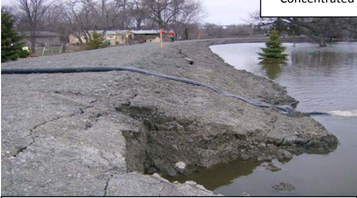
Scour from pump discharge hose.
