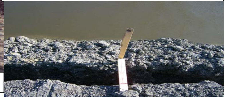
Monitoring of a levee crack.
