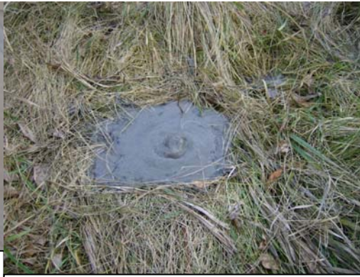
Concentrated seepage boil at levee toe.
