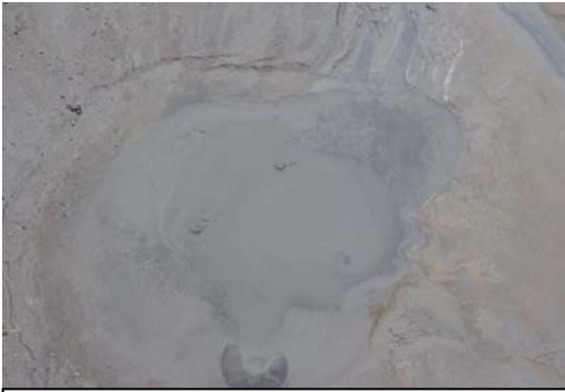
'Dirty' seepage carrying soil particles.
