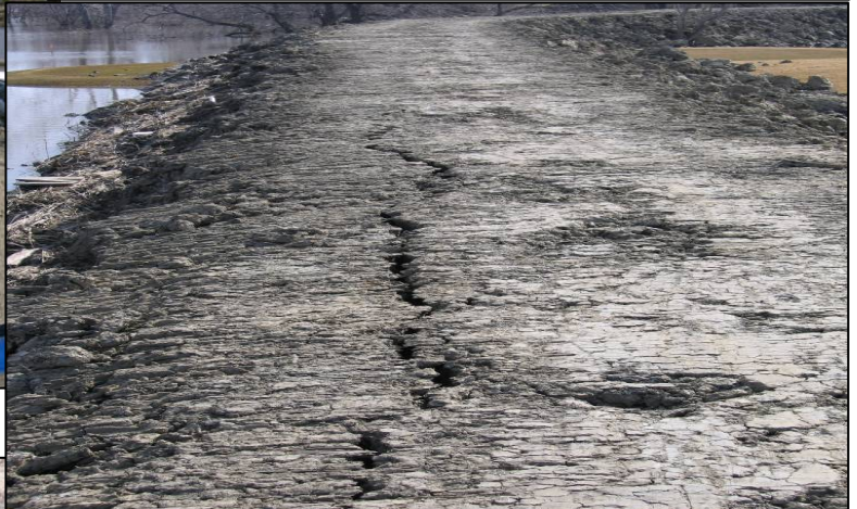
Formation of cracks along the levee.
