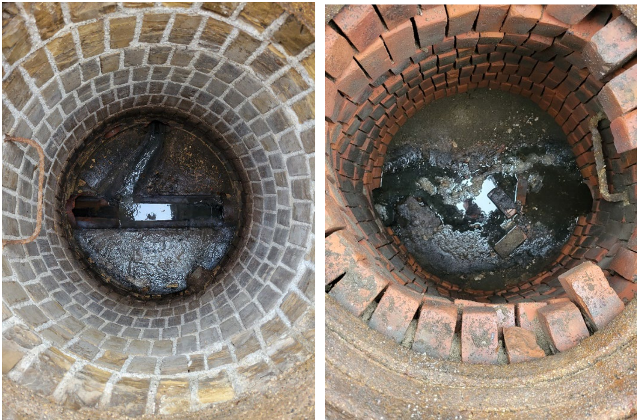
Figure 5. Sanitary Sewer Manholes: Fair Condition (Left) and Poor Condition (Right)
