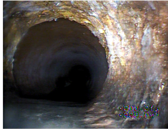
Figure 2: Transition from Cast Iron Piping to Clay Tile Piping – Unit 407W
