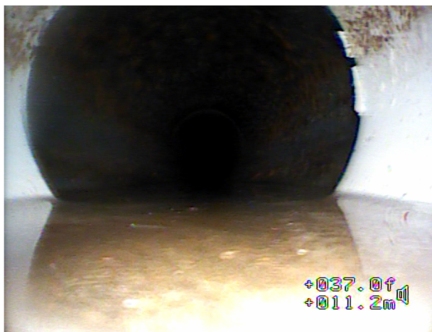
Figure 5: Transition from PVC to 3034 with Standing Water – Unit 412W
