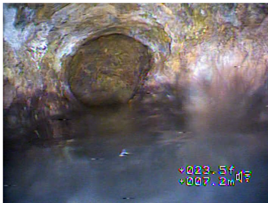
Figure 13: Corroded Cast Iron Piping and Standing Water within the Residence – Unit 413E
