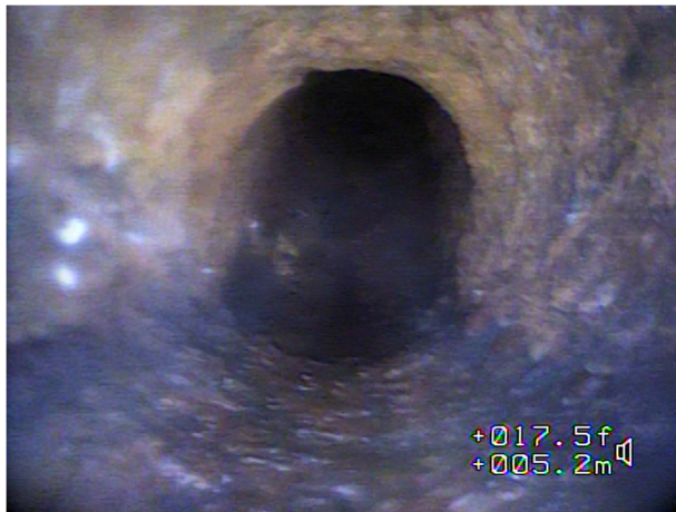
Figure 7: Corroded Cast Iron Piping within the Building – Unit 405E
