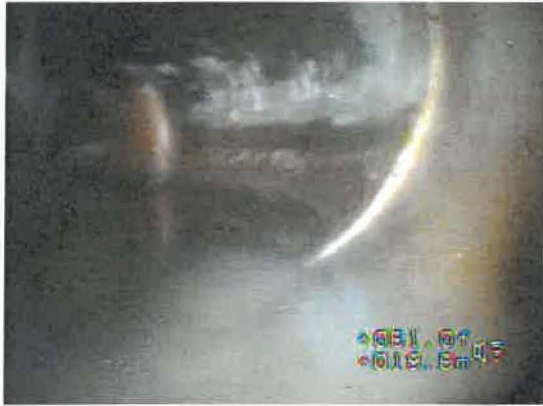
Figure 19: Standing Water and Fitting into Sewer Main – Unit 413E
