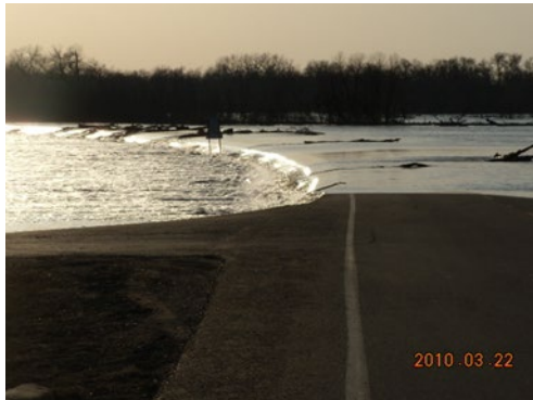
Spring flood flow over the emergency spillway at Lac qui Parle Dam on the Minnesota River.
